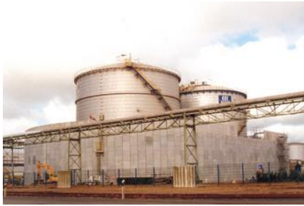
Containment dikes for ammonia tanks - Montoir (France)
